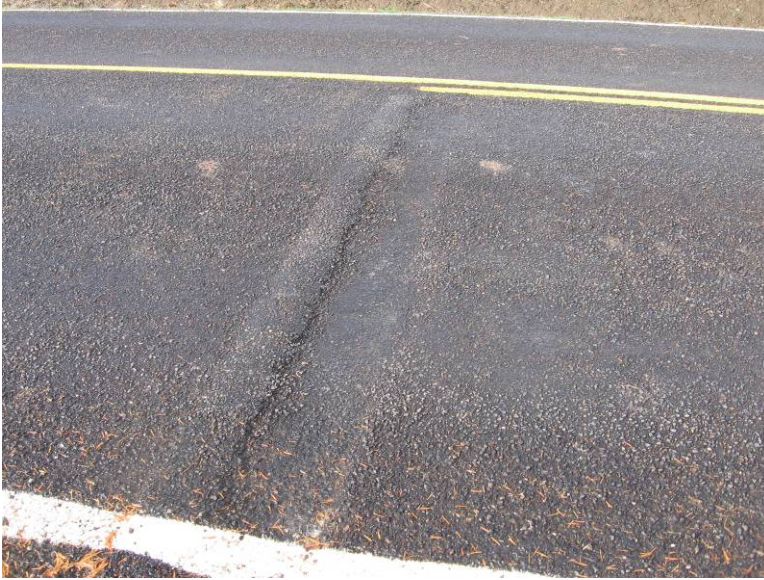
Transverse Joint improperly constructed.
