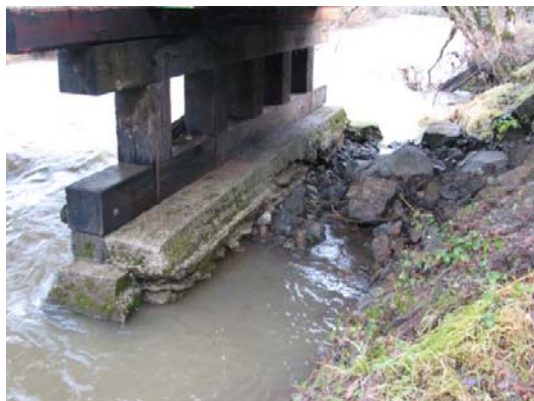
South Road (scour)
