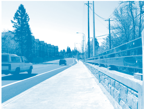
Cornelius Pass Road – Wilkins to Aloclek, including Rock Creek bridge replacement completed April 2013.
